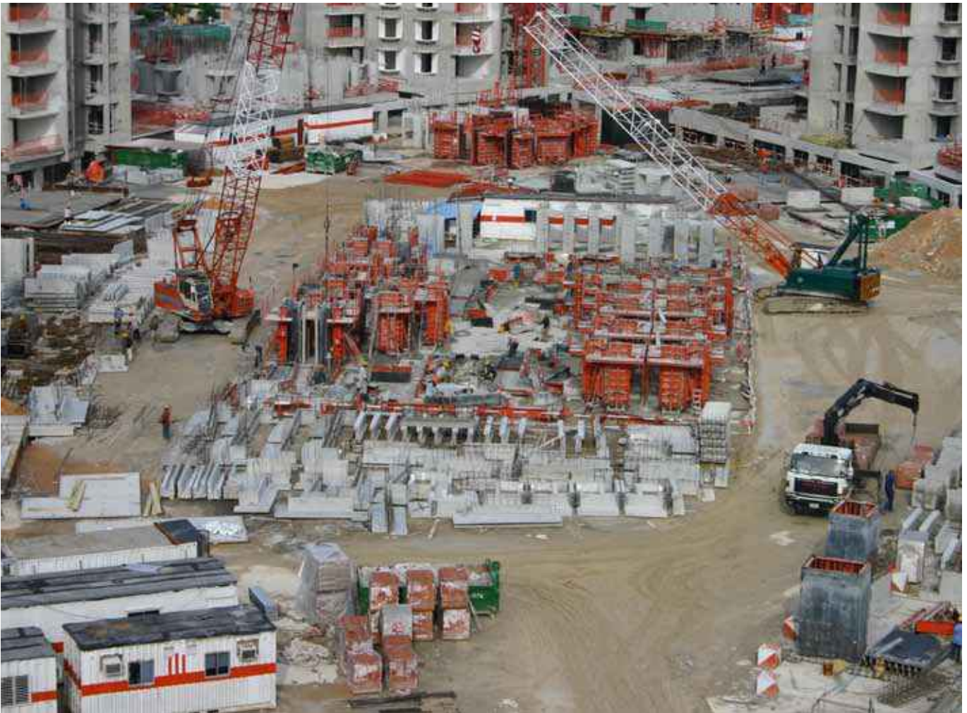
Above: An on-site pre-cast yard/factory like setting for the fabrication and storage of various pre-cast concrete building features of a given project.
