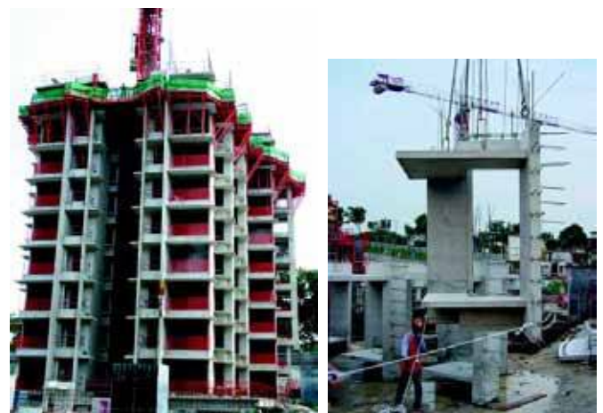
Above: Repetitive and complex corner features are being well integrated as pre-cast elements in the structure.
